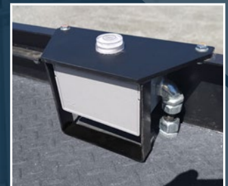
110v ac outlet on platform
